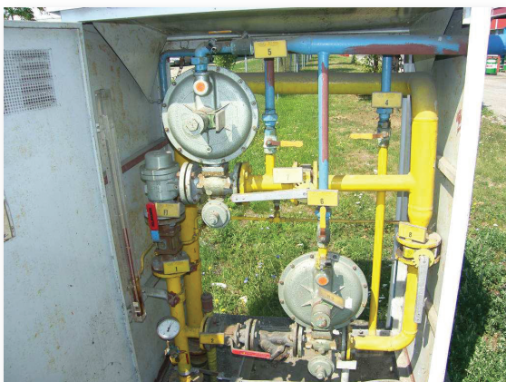
Gas pressure regulating station
