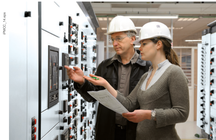
Motor Control Centre (MCC)
