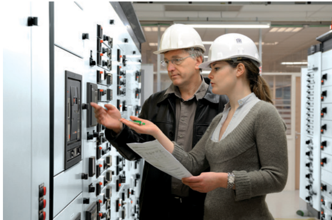
Motor Control Centre (MCC).
