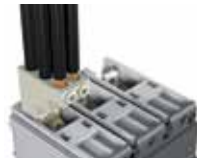
Multi-cable terminals with cables
