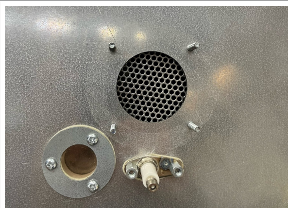
Figure 30 - The grid in front of the burner
