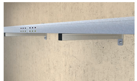
Cable duct on cantilever arm
