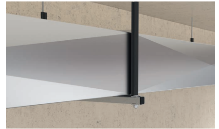
Ventilation duct fastening with suspended channel
