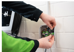
Connection of a wallbox / bicycle charging station
