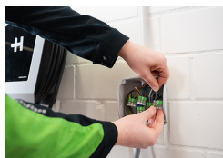
Connection of a wallbox / bicycle charging station
