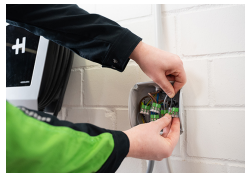
Connection of a wallbox / bicycle charging station
