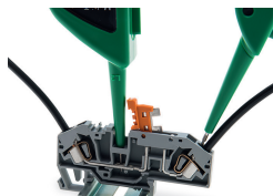
Testing via jumper contact slot.
