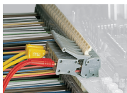
Testing with test plug modules.
