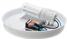
Connecting a light to the mains.
