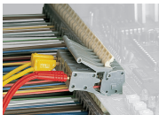
Testing with test plug modules.
