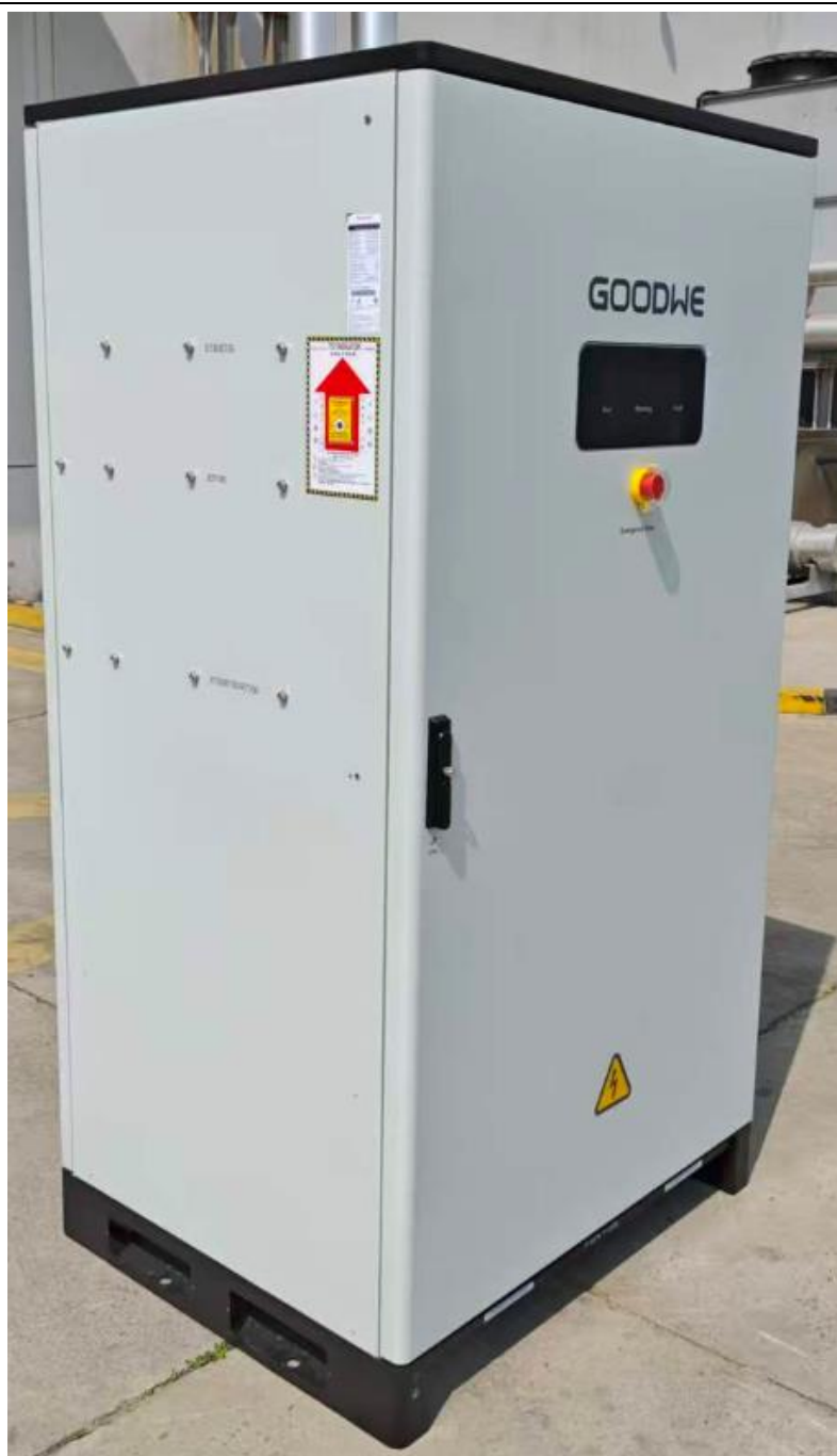
Figure 5a. Front view of battery unit
