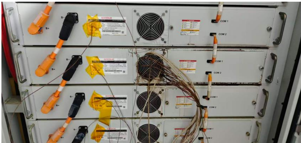
Figure 24. View of location of module that exhibited thermal runaway in the initiating unit
