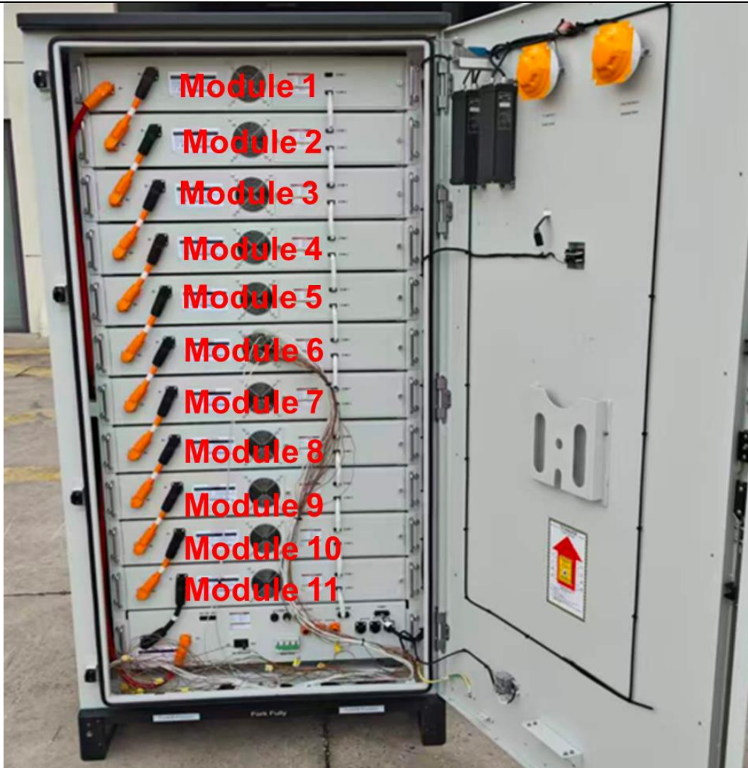
Figure 15. View of initiating module in BESS unit
