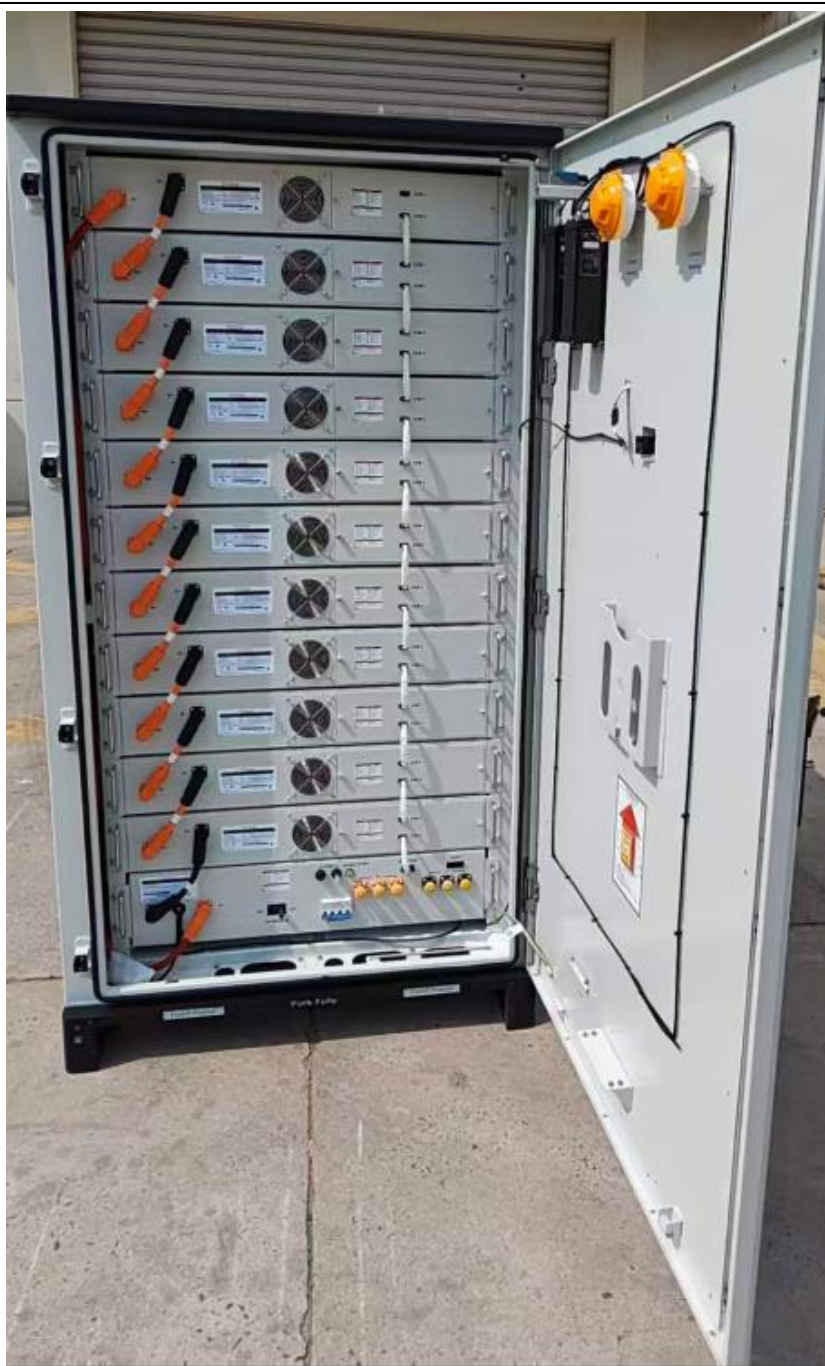
Figure 6. Internal view of battery unit (GW112.6-BAT-AC-G10)
