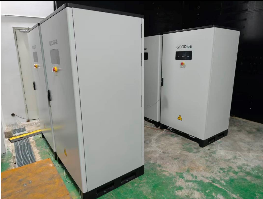
Figure 18. Front view of BESS units in testing room
