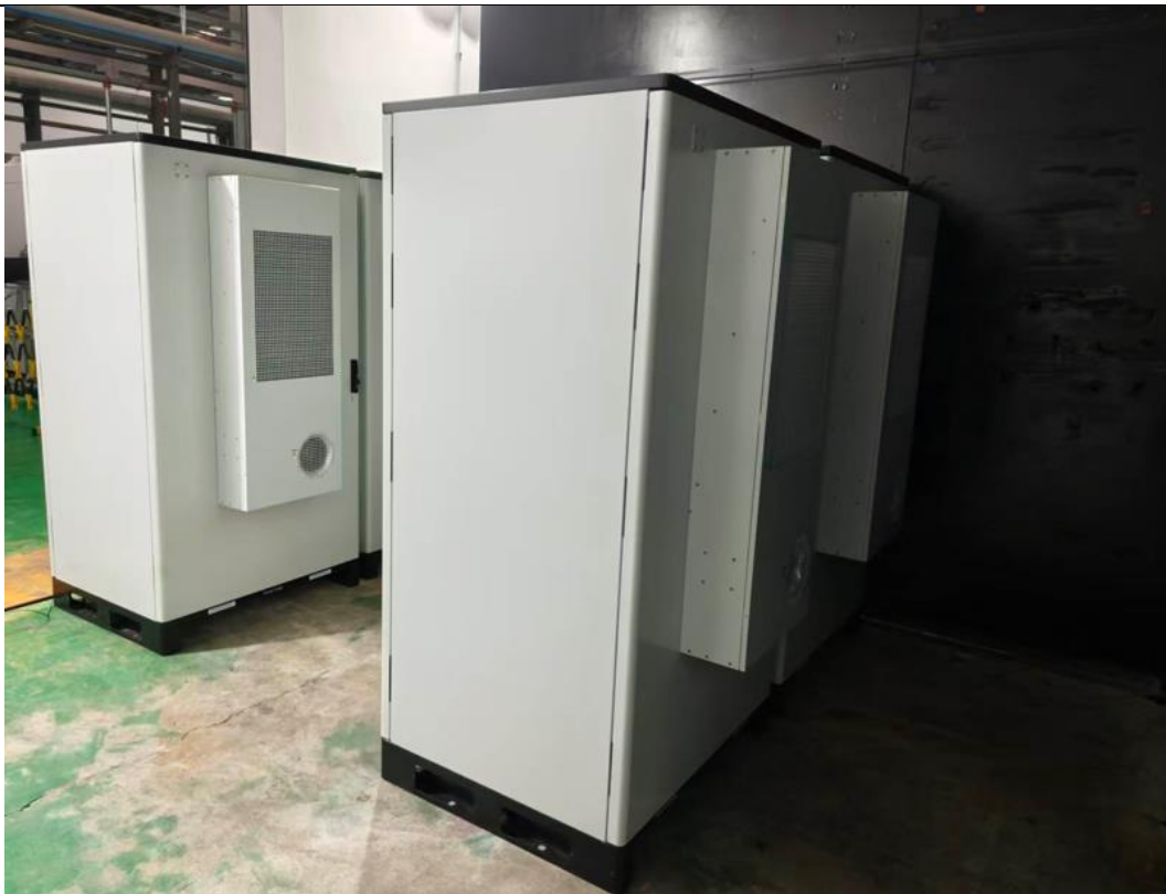
Figure 19. Rear view of BESS units in testing room
