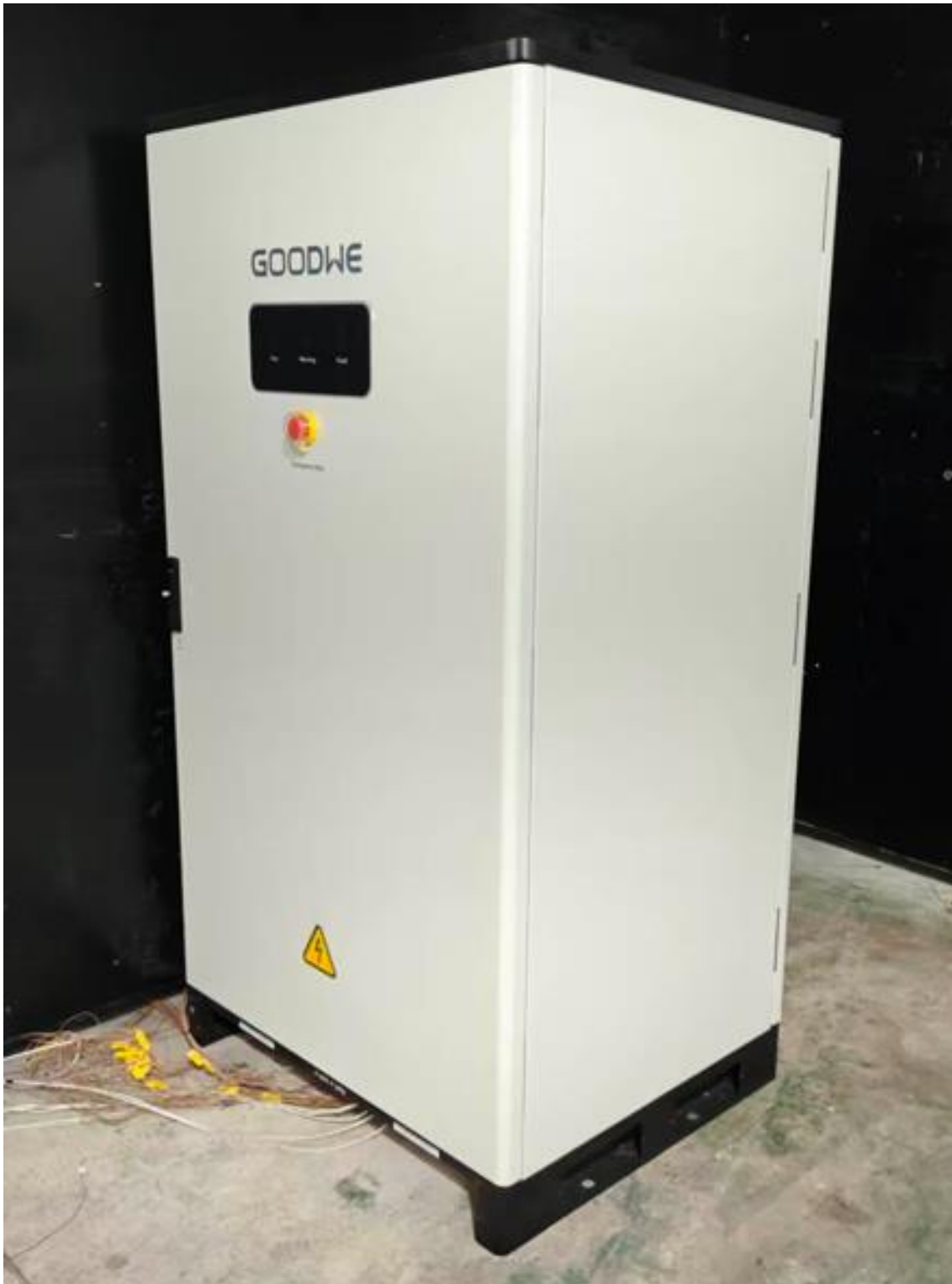
Figure 32. Photo of initiating BESS Units in testing room after test
